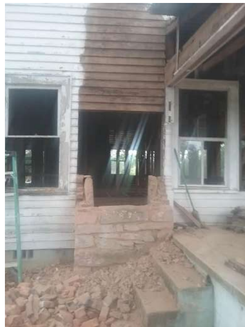
This photo shows the lower section of one chimney. All three chimneys have a granite base and firebox inside.
